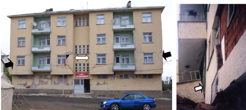
Fig. 1. Damage to Cantilevers due to the 2003 Bingöl Earthquake
