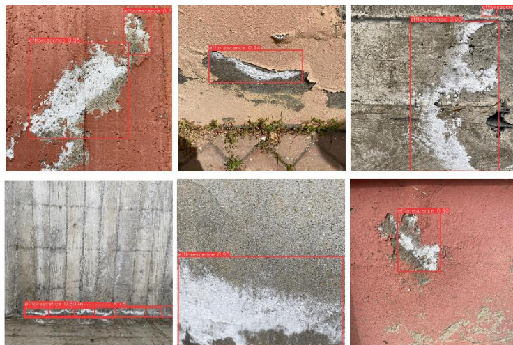
Fig. 7. Sample images of efflorescence detection
