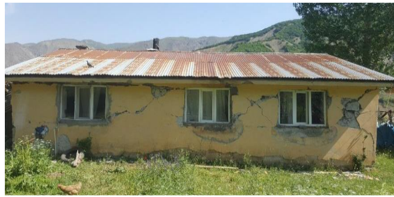
In-plan diagonal cracks [19]
