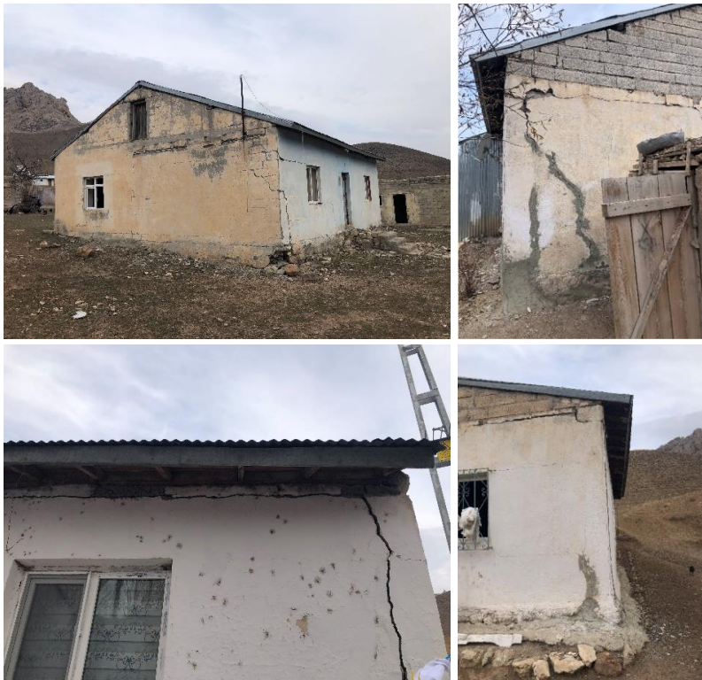
Fig. 10. Segregation damages at junction areas
