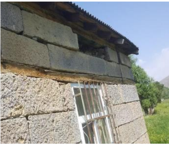
Poor wall-roof connection [20]
