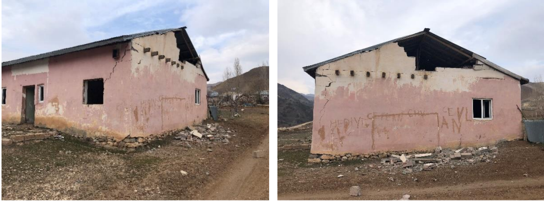
Fig. 9. Example of damage caused by poor connection between roof and walls
