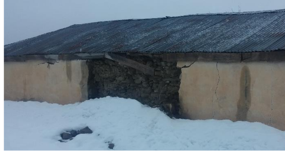
Out-of-plan wall collapse [19]
