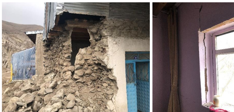
Fig. 11. Disconnection damage in multi-leaf walls
