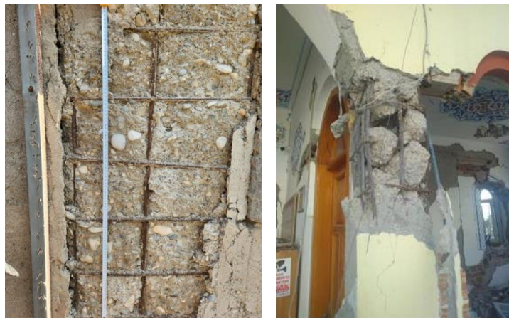
Fig. 11. Insufficient transverse reinforcement
