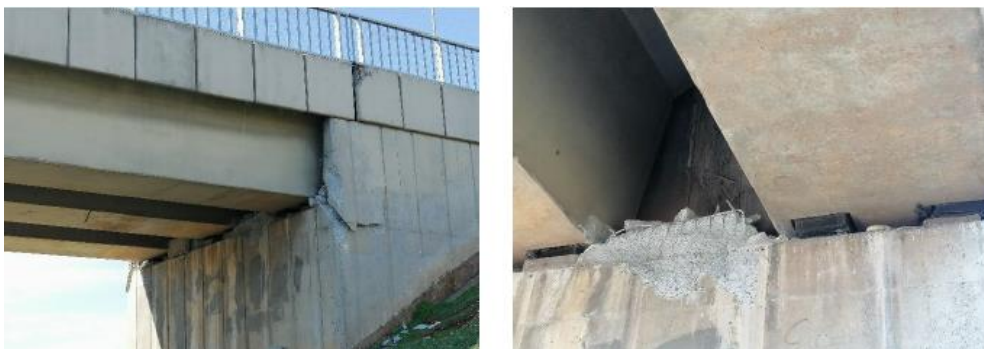
Fig. 22. The joint and support damages
