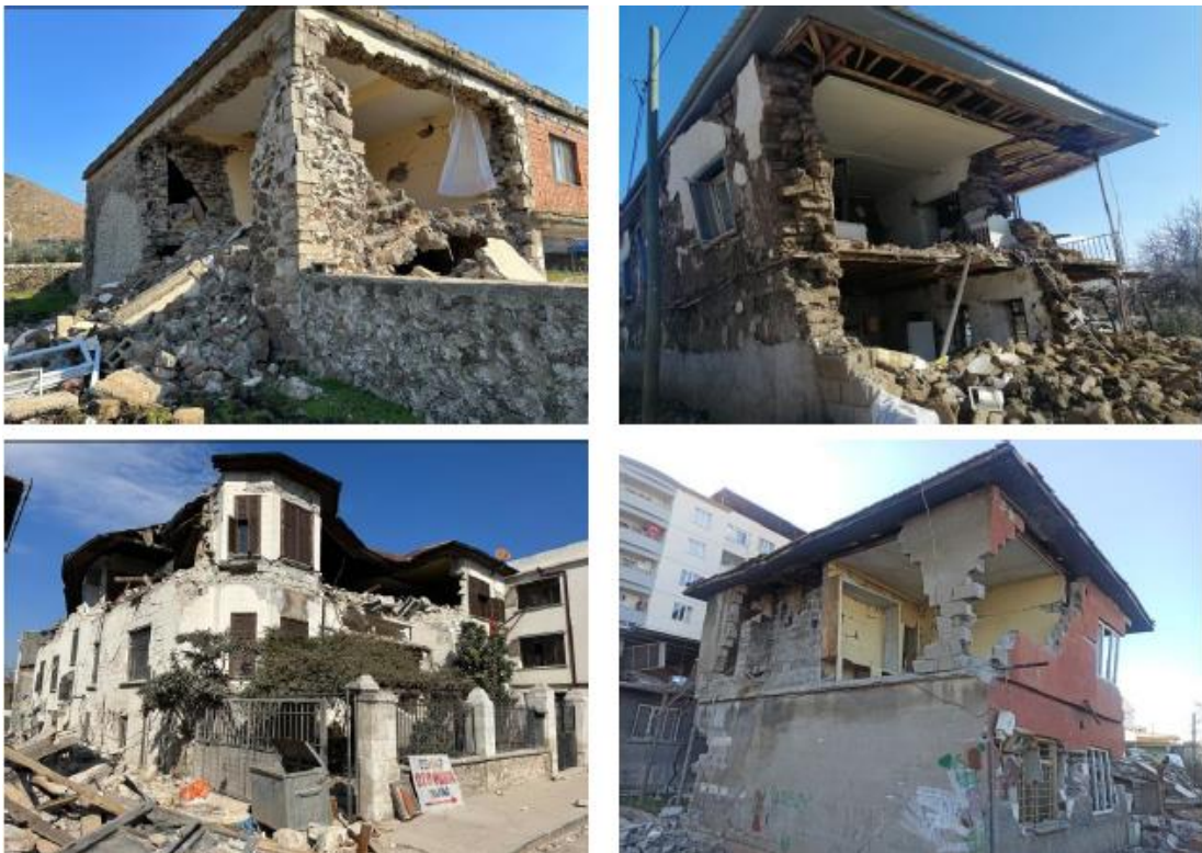
Fig. 18. Out-plane damages on masonry buildings
