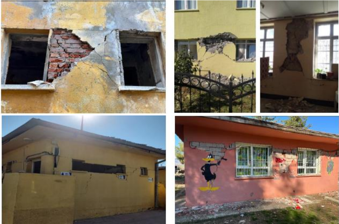
Fig. 17. In-plane damages on masonry buildings
