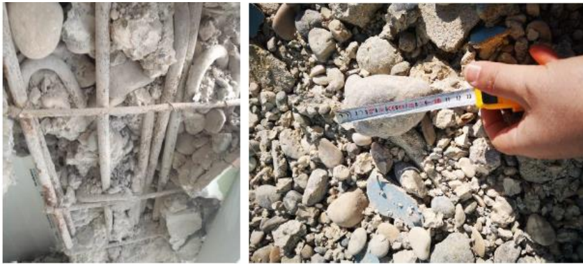
Fig. 14. Poor concrete quality
