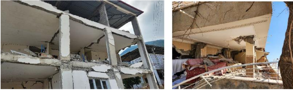
Fig. 12. Damages caused by hollow flooring application
