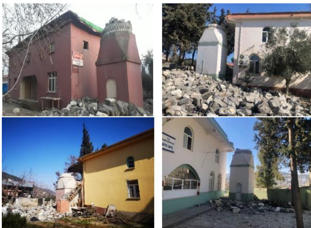
Fig. 28. Observed damages on reinforced masonry minarets
