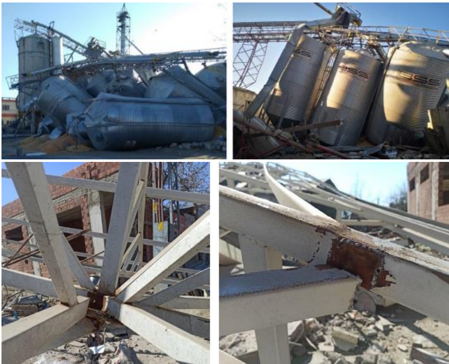
Fig. 19. The damages on steel industrial structures
