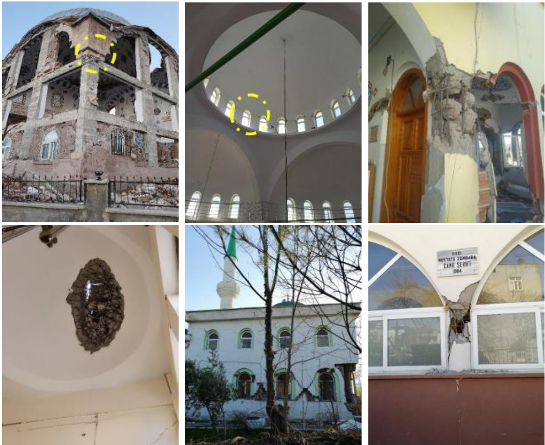
Fig. 25. Observed damages on reinforced concrete mosques
