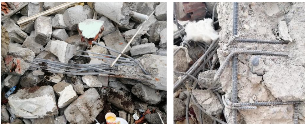
The incorrect placing of the reinforcement bar
