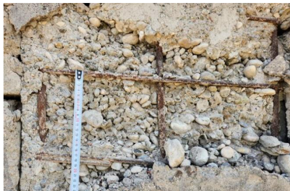
Fig. 15. Unribbed reinforcing bar and corrosion
