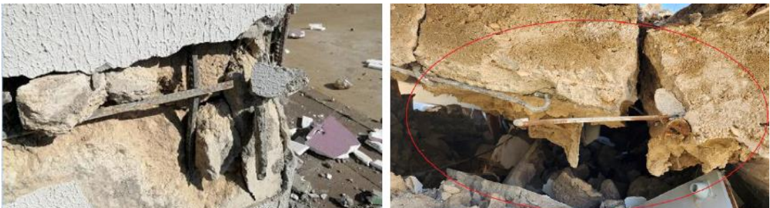
Fig. 9. Existence of short and unconfined lap splices
