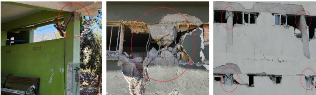
Fig. 7. Structural damage from short column formation
