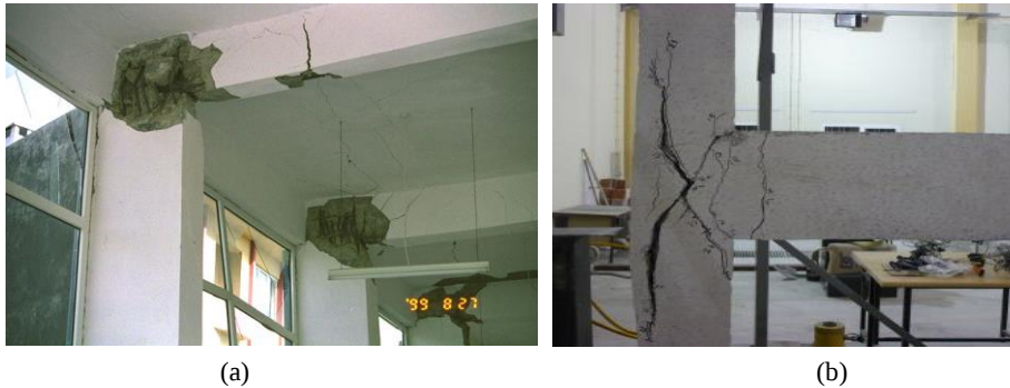
Fig. 1. Beam-column joint damages in (a) a residential building during 1999 Kocaeli Earthquake [8], and (b) a non-seismically detailed beam-column joint specimen [9]
