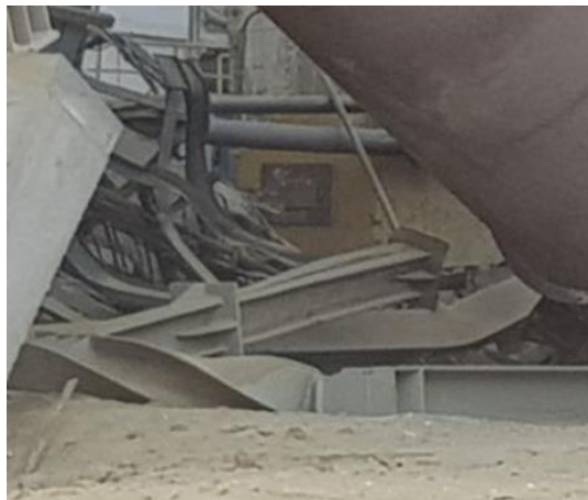
Fig. 18. View of the column after the collapse
