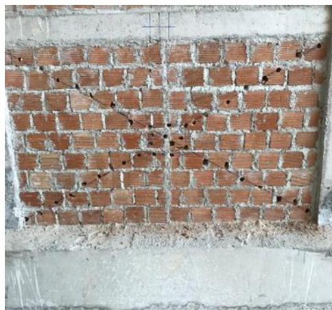
b) Detail view of damaged 1st storey
