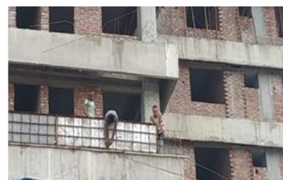
Fig. 9. Not using of PPE
