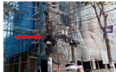
Fig. 7. No protection for street lamp, electric post
