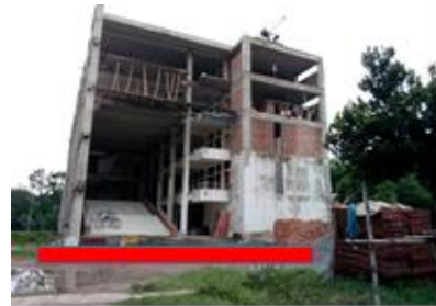
Fig. 6. No hoarding or barricade and safety sign provided
